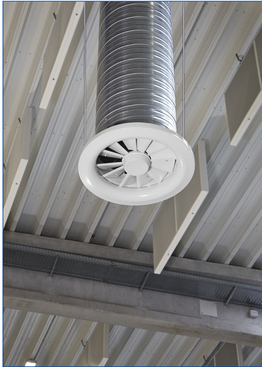
Freely suspended installation
